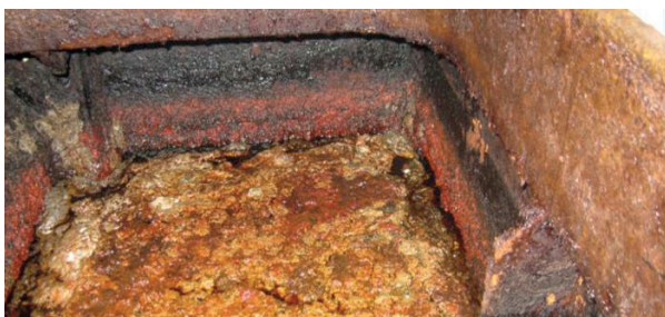
Existing issues with traditional treatment
