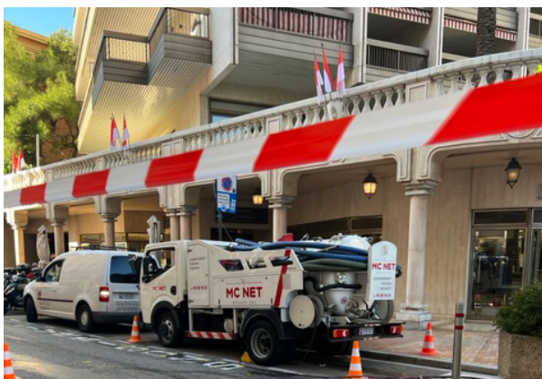
Truck sucking out fat and grease
